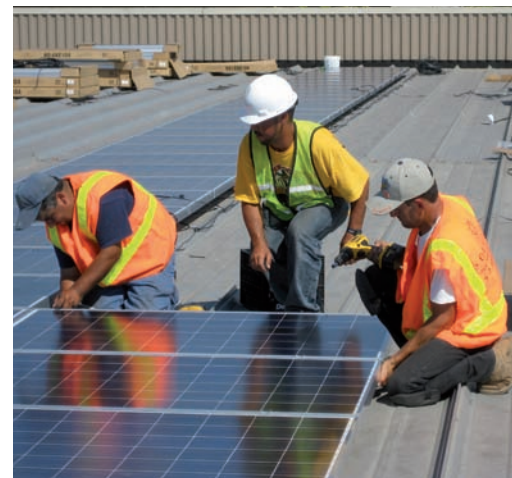
Solar panels provide 10 percent of residents' power needs PHOTO © BIOREGIONAL
