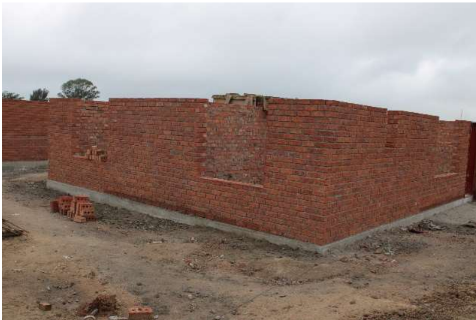
Source: Ministry of National Housing and Social Amenities archives. Construction of 7 x 4 storey blocks of flats in Senga, Gweru by the Ministry of National Housing and Social Amenities
