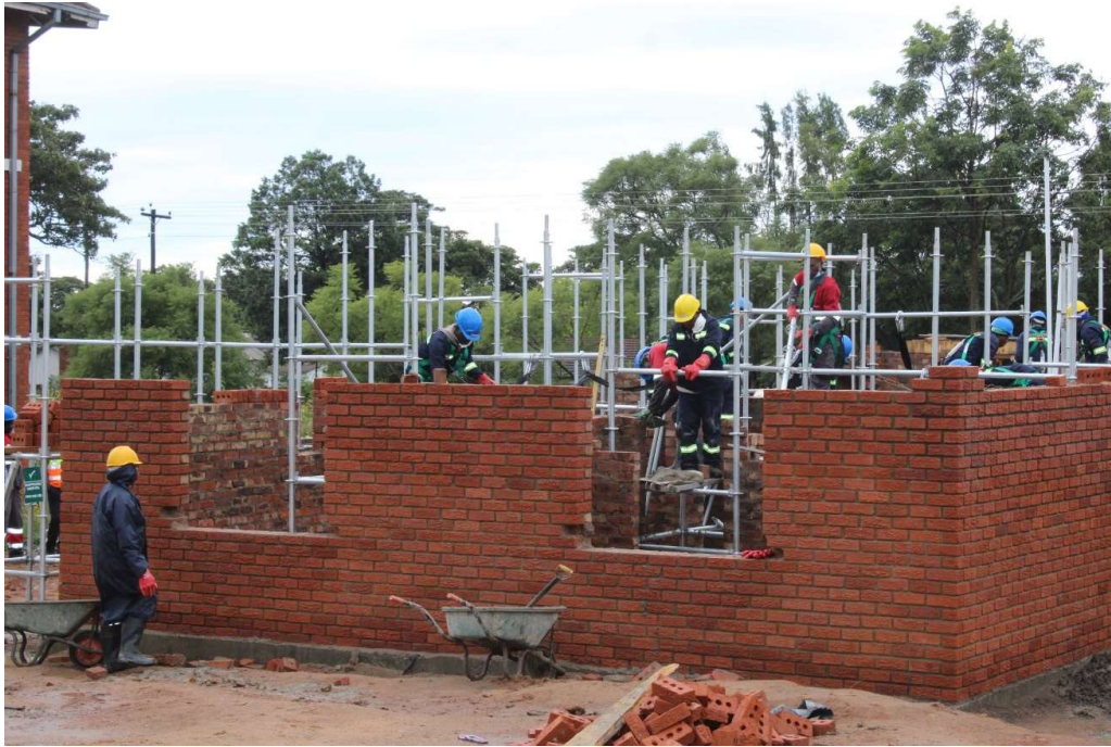
Source: Ministry of National Housing and Social Amenities archives: Construction of 4 x 4 storey blocks of flats in Marondera by the Ministry of National Housing and Social Amenities
