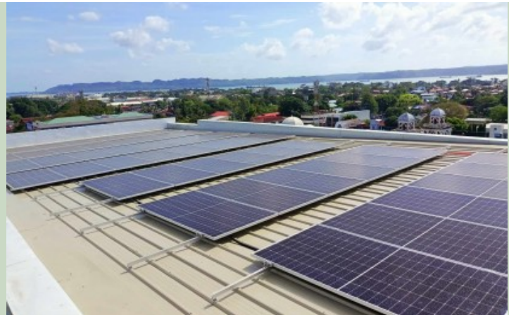
Iloilo City Government installed 134 solar panels atop the City Hall. The solar panels are expected to generate 60 kilowatts a day and will cover around one-third of the power demand at the City Hall Photo from Philippine News Agency, January 15, 2024
